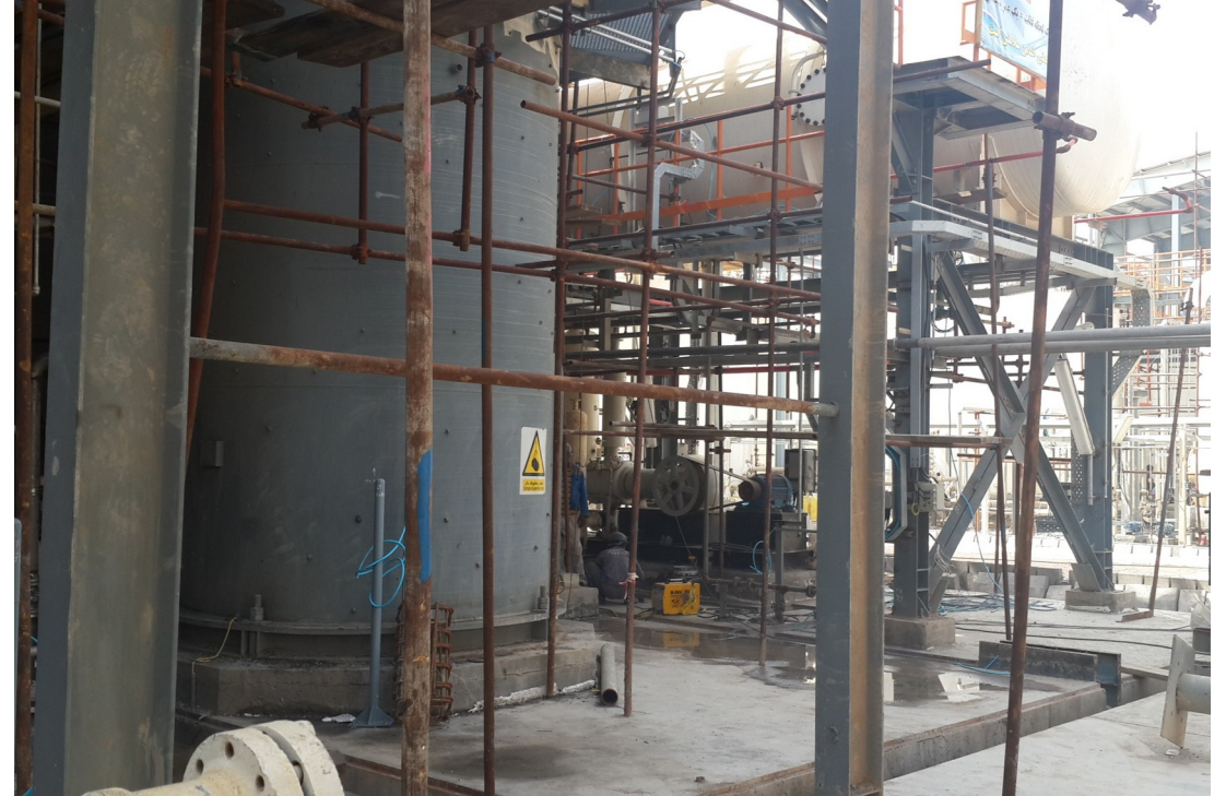
Equipment and field engineering
